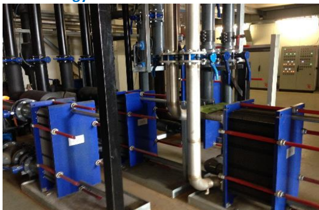
Fig. 3 Plate heat exchangers as part of an ATES system
