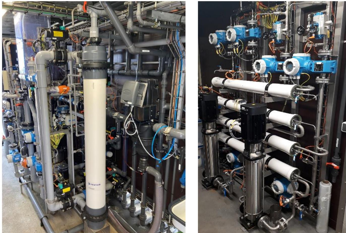
Fig. 4 Pilot plant in Kalundborg (from left to right): UF module, RO units
